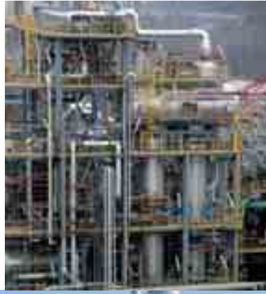
Boiling reactor at LVM, Tessenderlo, Belgium 250,000 t/year of EDC
