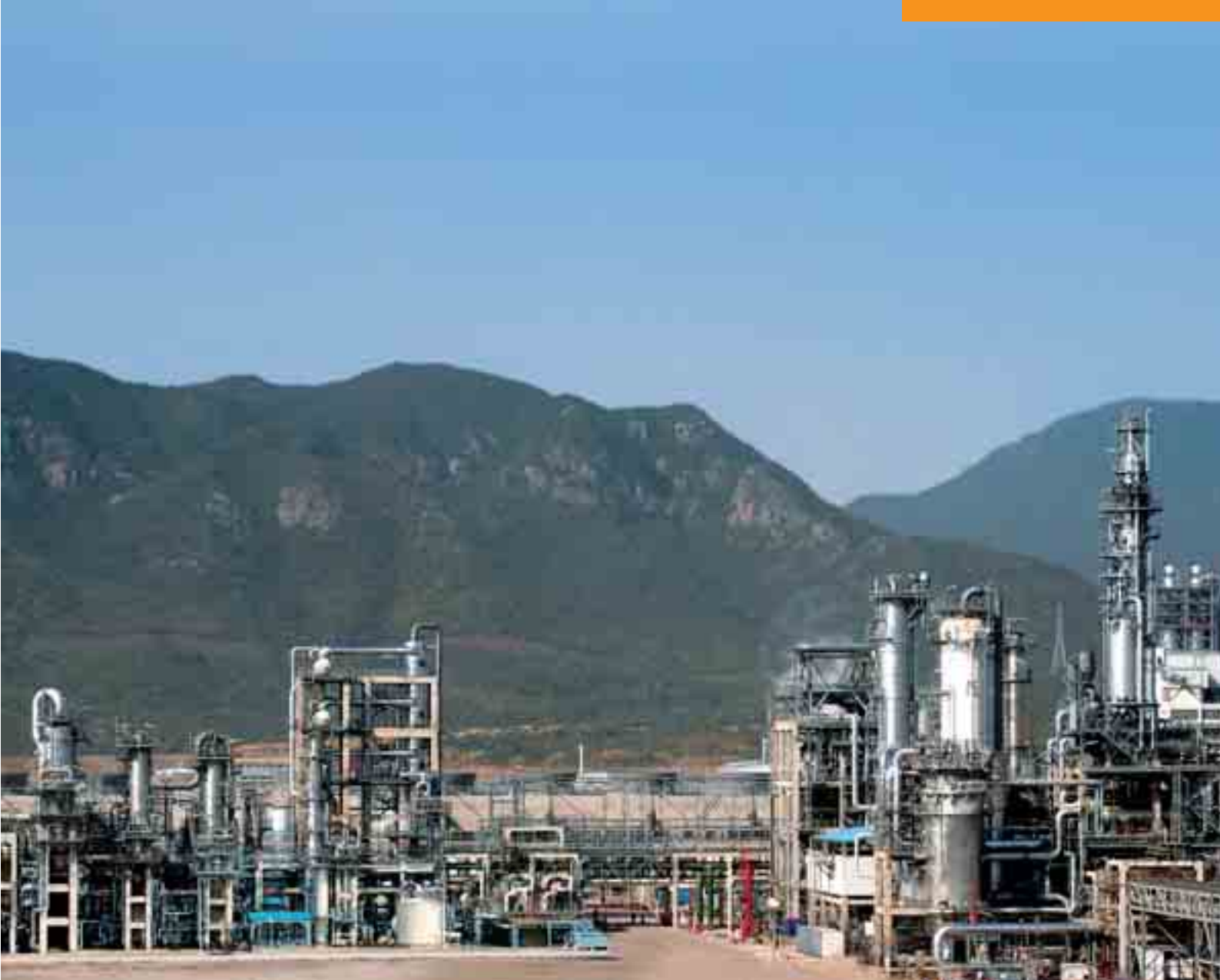
CNOOC / Shell Nanhai Petrochemical Complex, China EO/EG plant: 320,000 t/year of mono ethylene glycol
